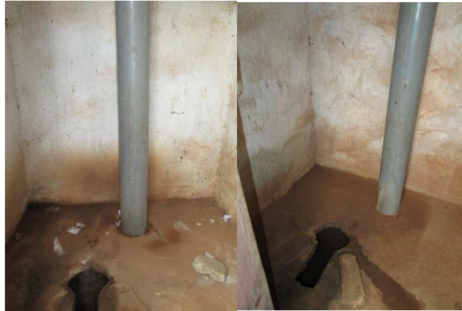
Figure 15 JVS Boys' Latrine (left) and Girls' Latrine (right)
